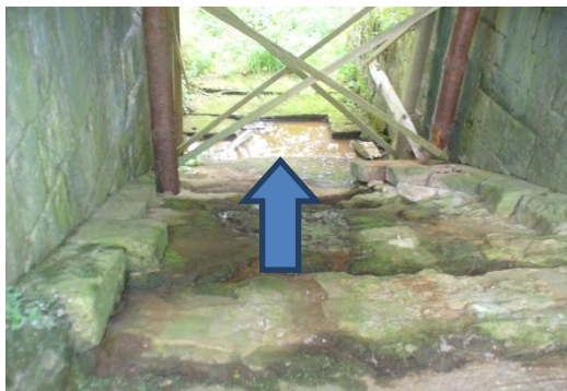
Southern Spillway – stone removed by storm water
