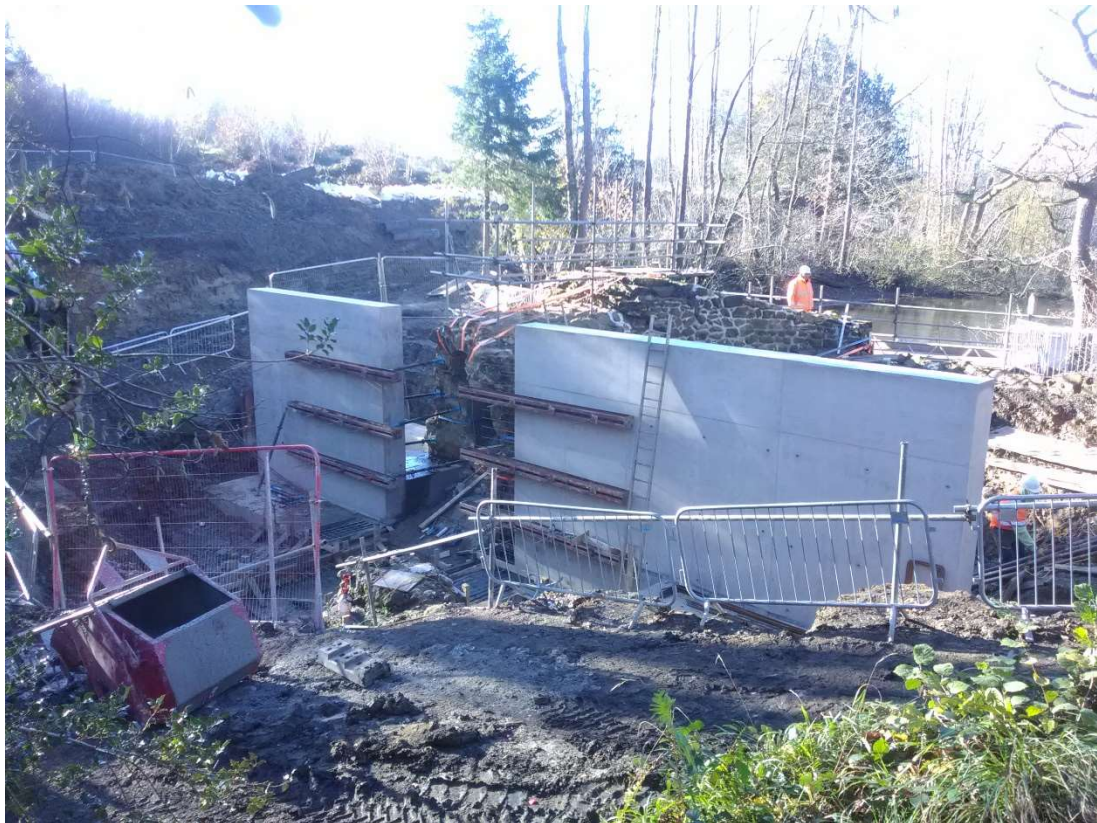
The second piece of concrete wall is 8 m long and used 13 cu m of concrete
